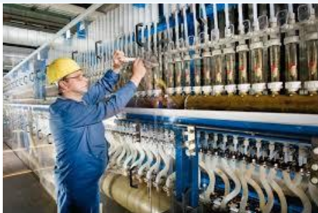
Electrolysis cell hall
